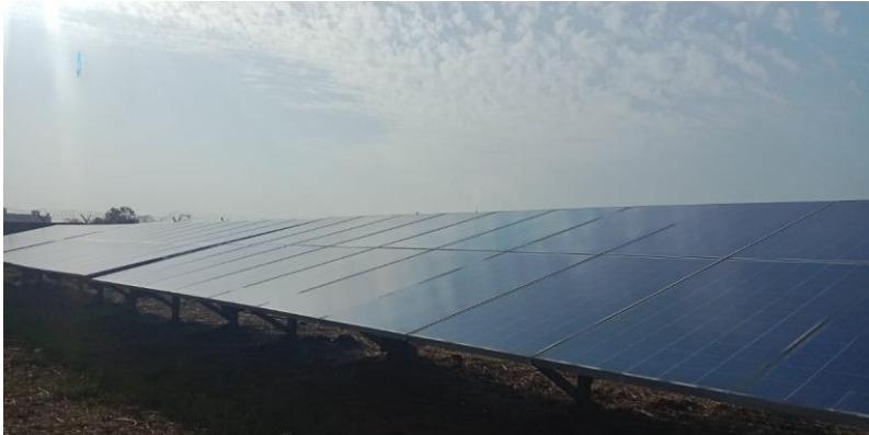
1 MW captive solar power plant, generated power used in construction activity
