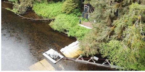
(b) Koeye River weir setup and solar panels
