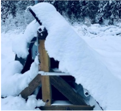
(c) Solar panels in the harsh winters of Bear Creek River
