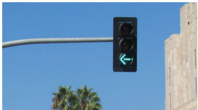
Left Turn Signal Phasing provides a green arrow for left turning vehicles while stopping conflicting vehicles and pedestrians.
