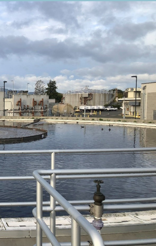
Photo to left: Secondary clarifier at Novato Sanitary District's wastewater treatment plant, covered under a NPDES permit
