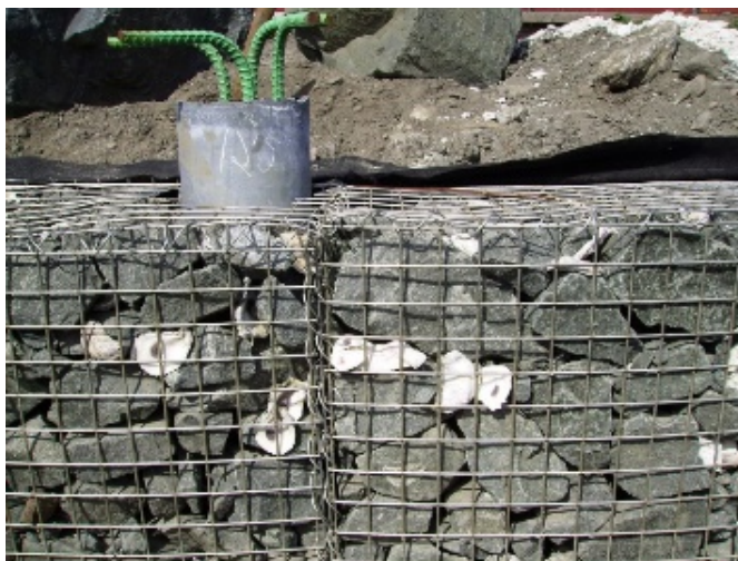
Figure 9: Gabion baskets used at Harlem River. Source: https://harlemriverpark.weebly.com/gallery.html Photo by: Thomas Lunke
