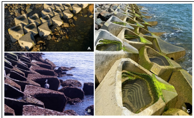
Figure 18: Pilot Project Installation on deployment day (A), eight months post construction (B), and three months post construction (C).
