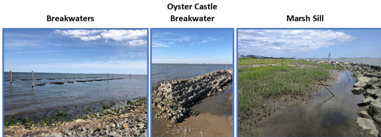
Figure 1: Example Living Shorelines Projects (From left to right: breakwaters, an oyster castle breakwater, and a marsh sill)
