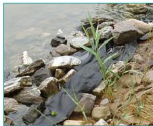
Filter fabric beneath rock footer. Photo credit: Alison Ward-Maksym, NOAA Restoration Center
