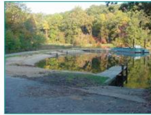
Completed site: post-bulkhead removal, shore regrading, and replanting. Photo: Rich Takacs, NOAA Restoration Center
