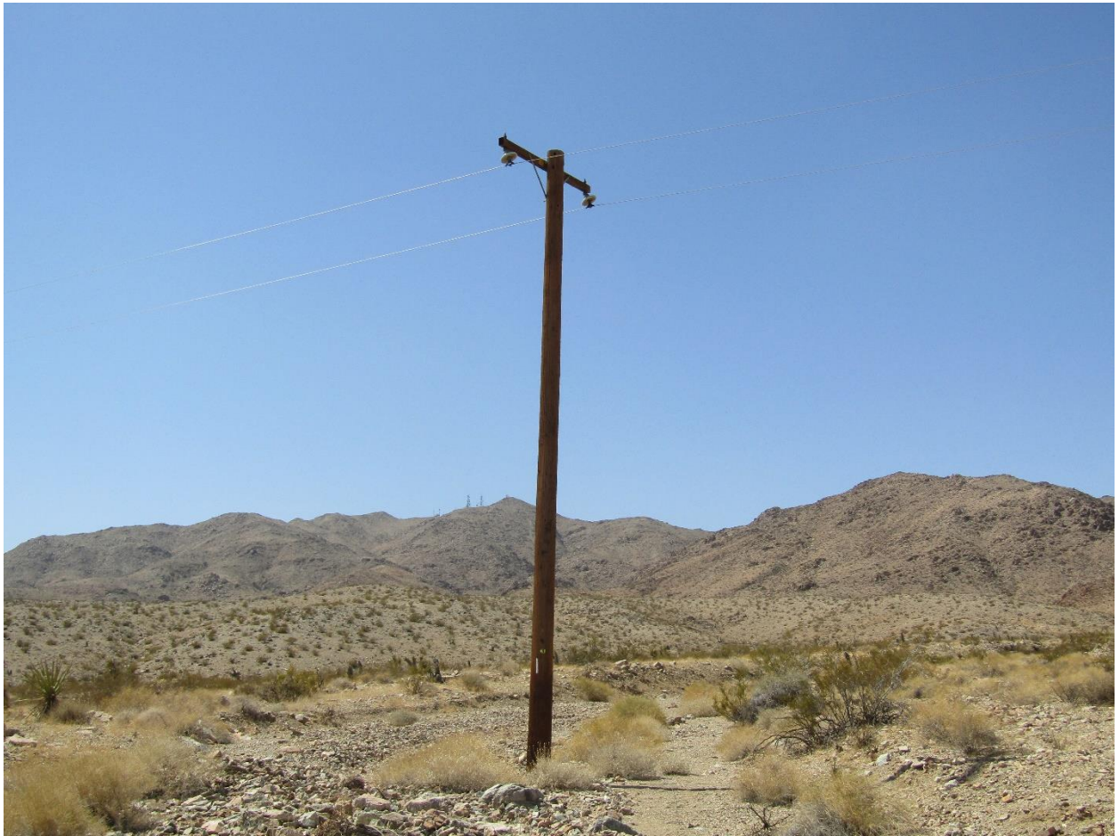
Figure 4: Overview of Pole 1977202E and drainage feature. Photo is facing upstream (northwest).
