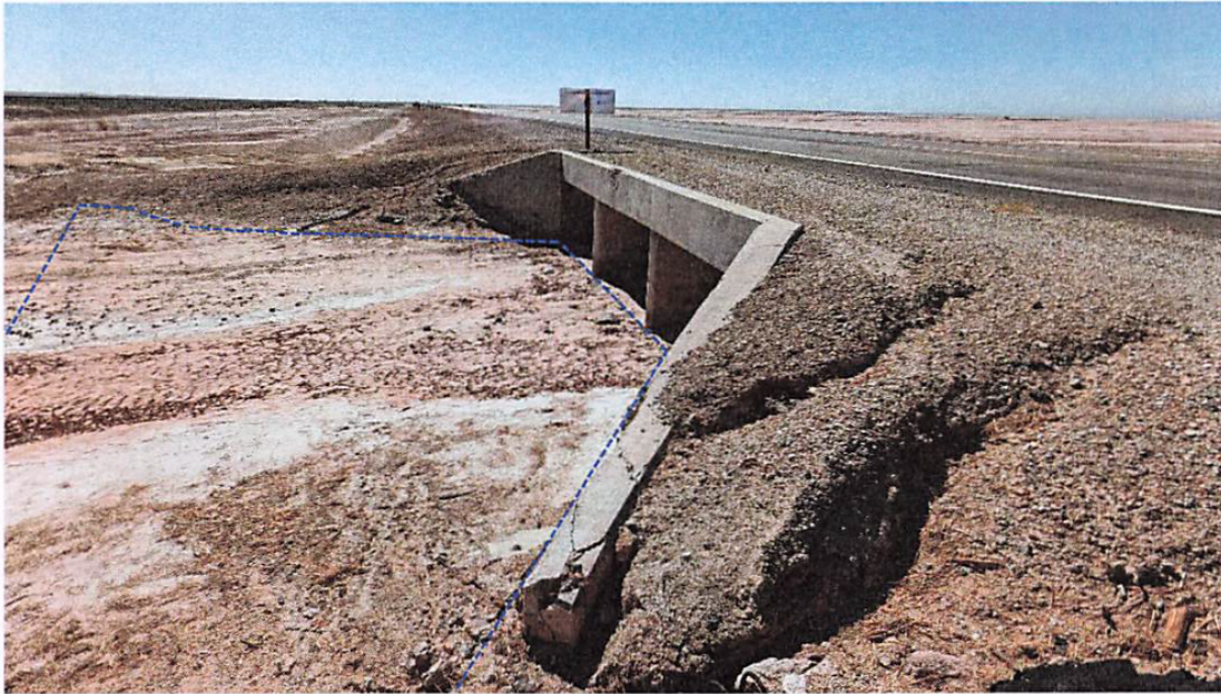
Photo C2. Imperial County, SR 111, PM 50.65 at Clay Wash. Proposed staging area upstream of the roadway, view southeast at the south bank.
